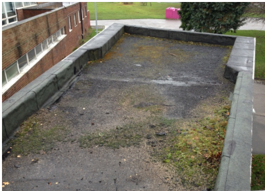
Debris and flat roof condition to entrance canopy roof area 1.
