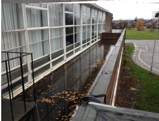
Significant ponding to flat roof area 3.
