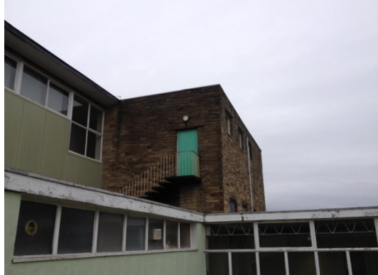
Elevation E10A, repairs recommended repairs not carried out. Loose stonework to corner needing repair.
