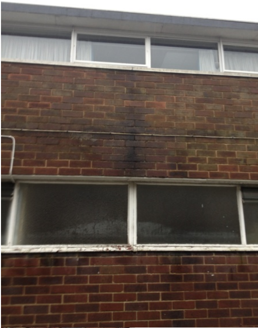
Leakage through brickwork due to ponding on roof area 3.
