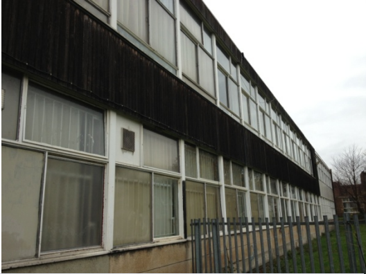
Elevation showing general degradation typical of the perimeter.
