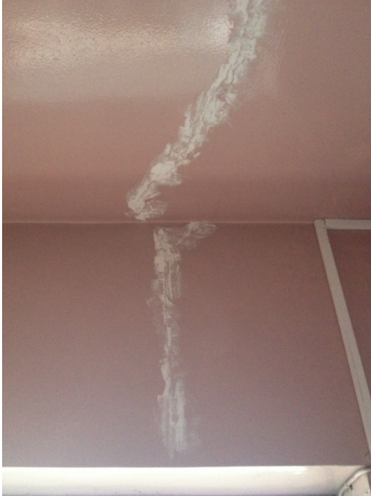
Office areas G224-232. Example of cracking to soffit with evidence of potential continuing movement.
