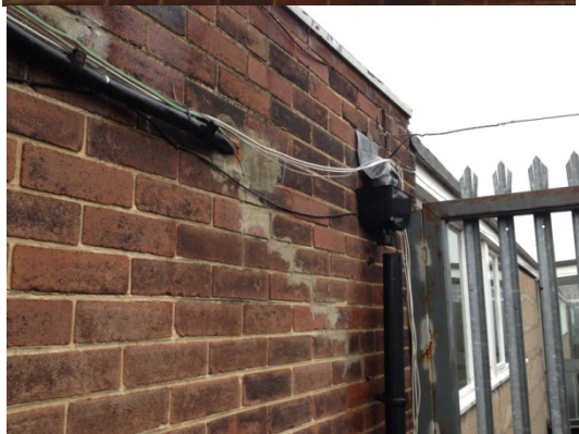
Cracking to NW end of roof 2, no elevation reference showing potential evidence of continuing movement.
