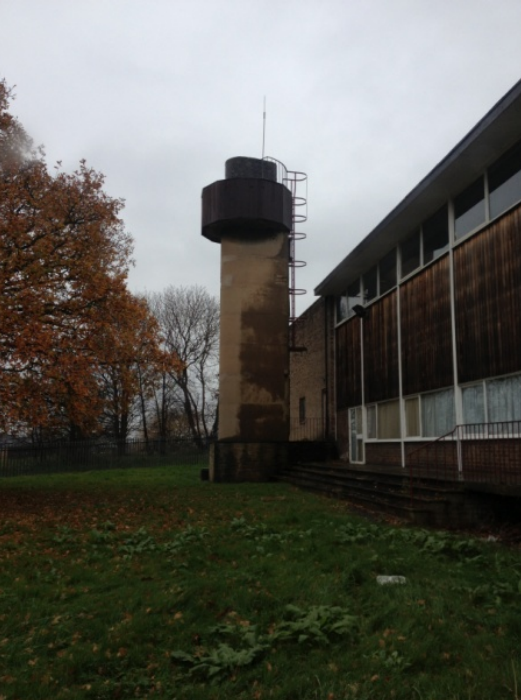
Spalling and degradation to water tower, section loss and exposed rebar. Elevation E6.
