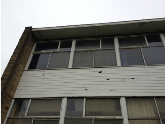
Deterioration and damage to cladding and soffits elevation E24.
