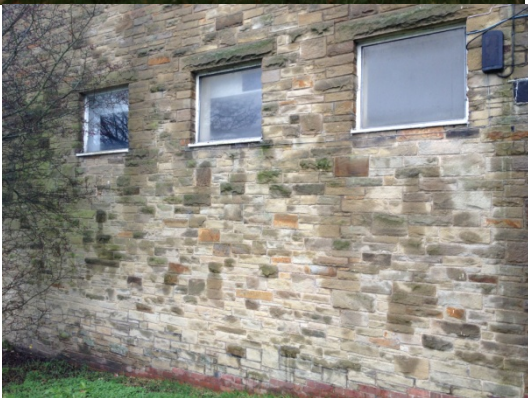
Cracking to Ashlar wall. Potentially settlement.
